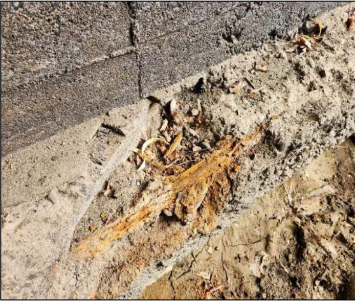
Fig 8: Localized concrete failure and rebar corrosion
