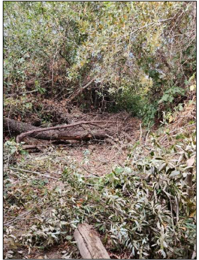
Fig 13: Tree trunk and debris downstream within channel
