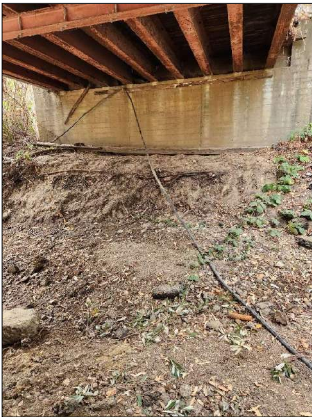
Fig 10: Unknown black cable disappearing underground at South abutment.
