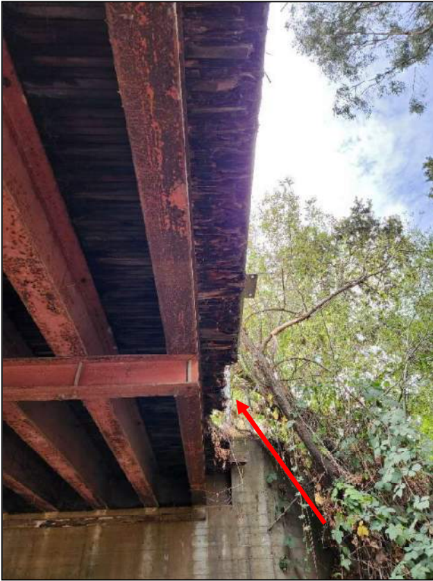
Fig 20: Timber decking deterioration on Southwest edge of bridge
