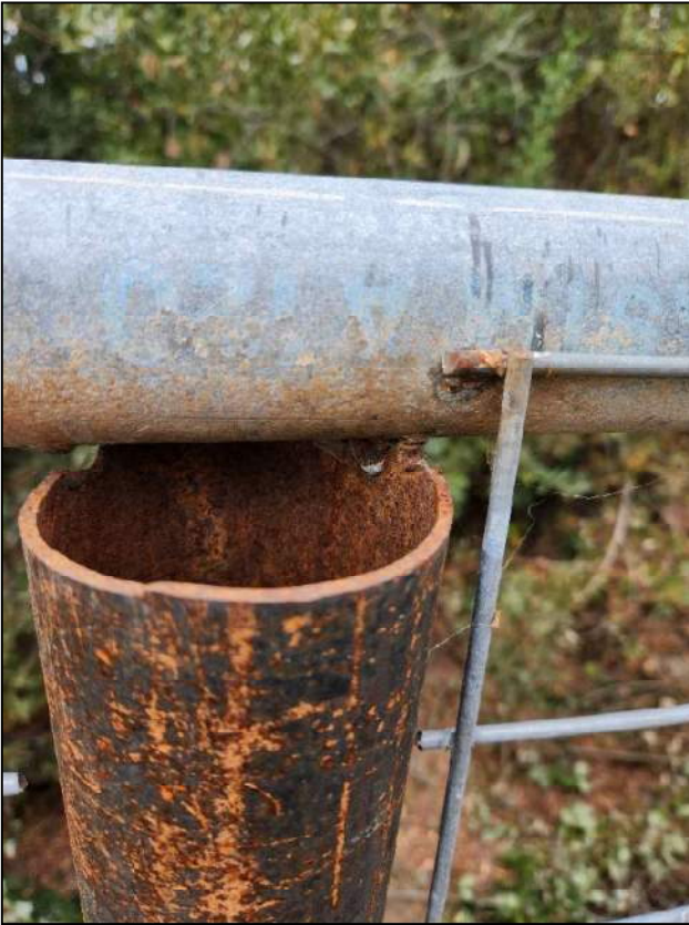
Fig 24: Tack welds holding railing together
