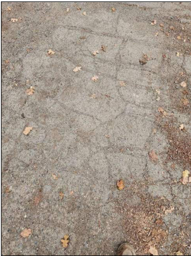
Fig 26: "Alligator" cracks at approach
