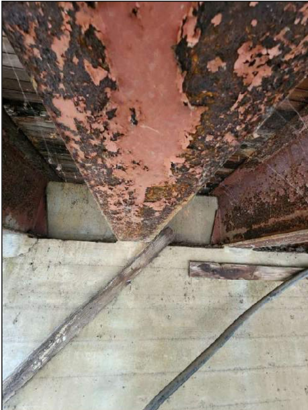
Fig 18: Paint peeling off from steel girders
