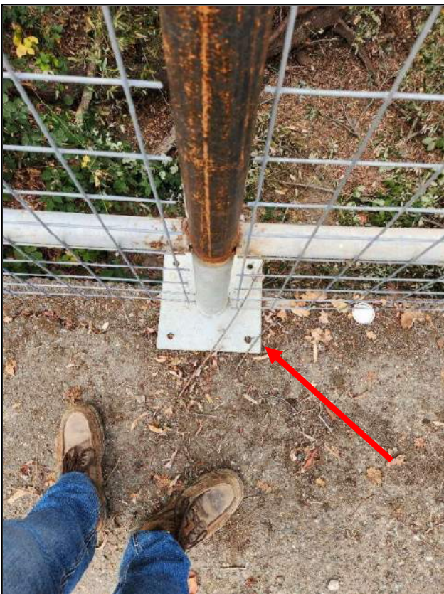
Fig 22: Post not attached to any part of deck
