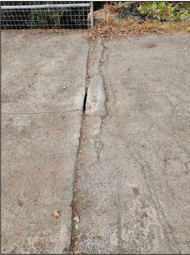
Fig 28: North abutment crack at expansion joint
