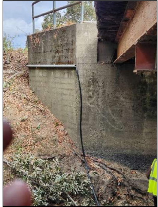
Fig 6: Northwest wingwall with metal conduit and cable
