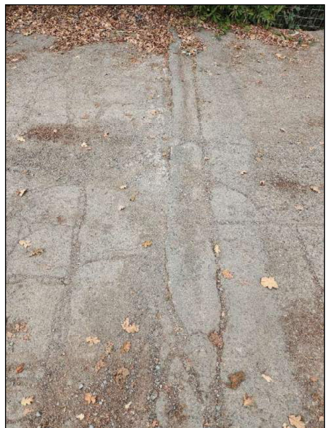
Fig 27: South abutment crack at expansion joint
