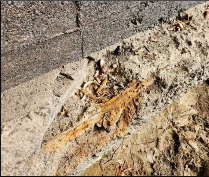
Fig 8: Localized concrete failure and rebar corrosion
