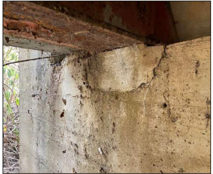
Fig 9: "Intact" spalling at South abutment bearing
