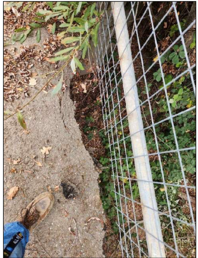
Fig 21: Asphalt crumbling on Southwest edge of bridge
