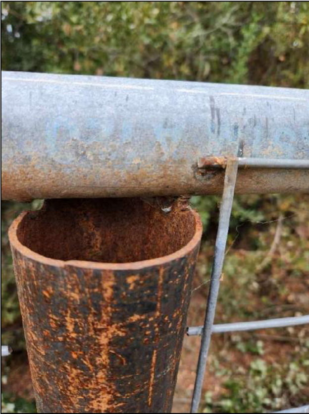
Fig 24: Tack welds holding railing together
